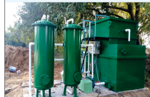
Sewage Treatment Plant
